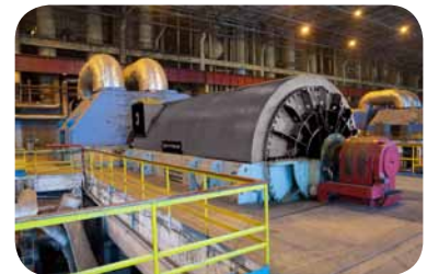
Skoda Power used Optimus to achieve 16% reduction in stress peak values steam turbine blades. The average stress in sensitive blade regions and the contact pressure between rotating parts also decreased.
